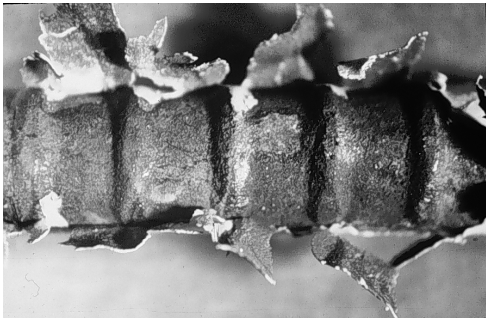
(c) Corrosion on bar from cracked loaded beam B11
