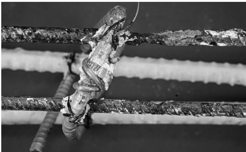
(b) Severe pitting on black bars near coated stirrup (beam B23)
