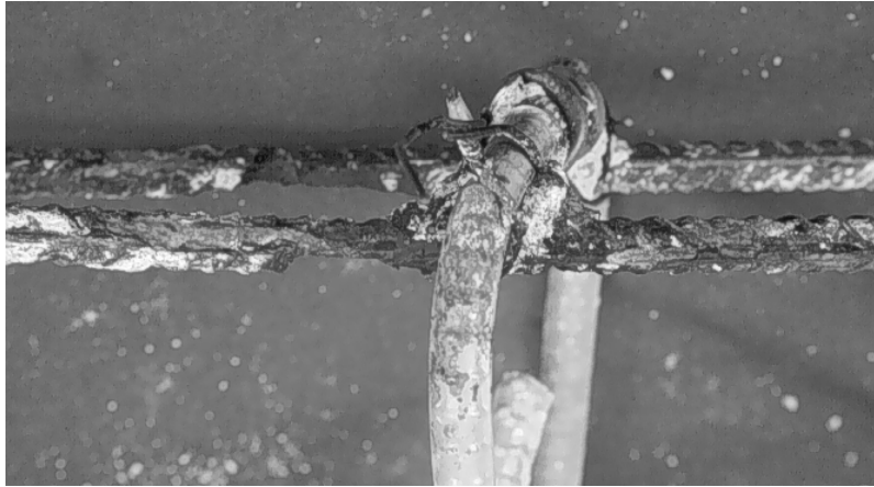
(a) Severe pitting on lower black bar near coated stirrup (beam B23).
