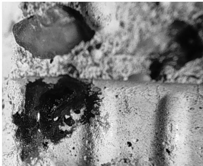
Figure 2.44 Corrosion spots coincident with voids in concrete (specimen removed after one year).
