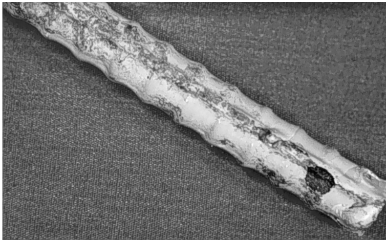
Figure 2.54 Corrosion on hook end of stirrup removed from cracked loaded beam after one year of exposure.
