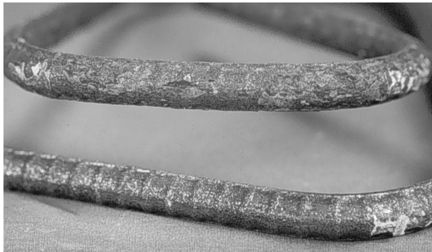
Figure 2.85 Corrosion on stirrup leg (top in photo) and mottled surface on stirrup hook (bottom in photo). Portion near the front beam surface (beam B32).
