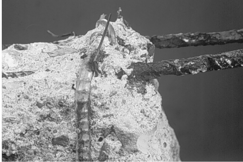
Figure 3.9 Pitting corrosion of uncoated bars at crack location (beam B25).
