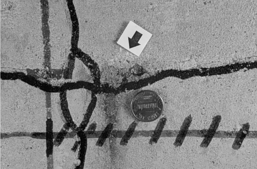
Figure 2.40 Rust exuding through cracks on front surface of beam B32.
