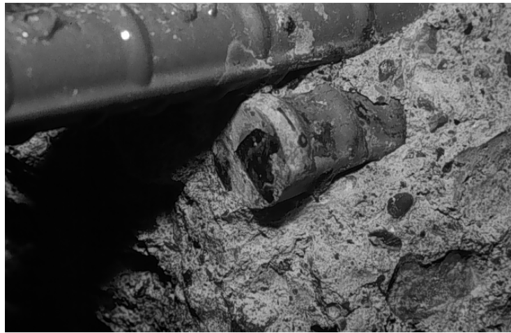
(b) Lower splice bar, appearance of bar end at time of autopsy
