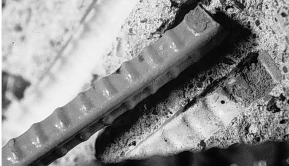
Figure 2.90 Patching material observed on stirrup imprint in concrete.
