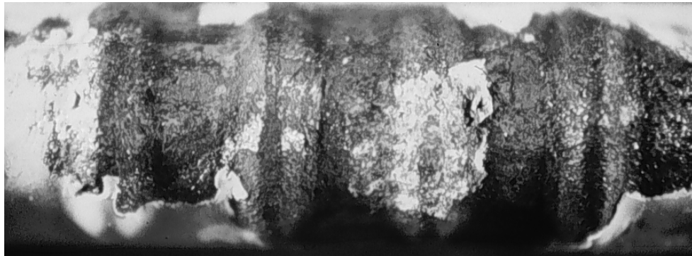
(b) Corrosion on bar from cracked unloaded beam B9
