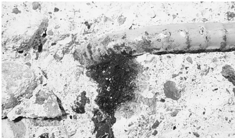
Figure 3.26 Corrosion at location of contact of coated stirrup and uncoated bar.
