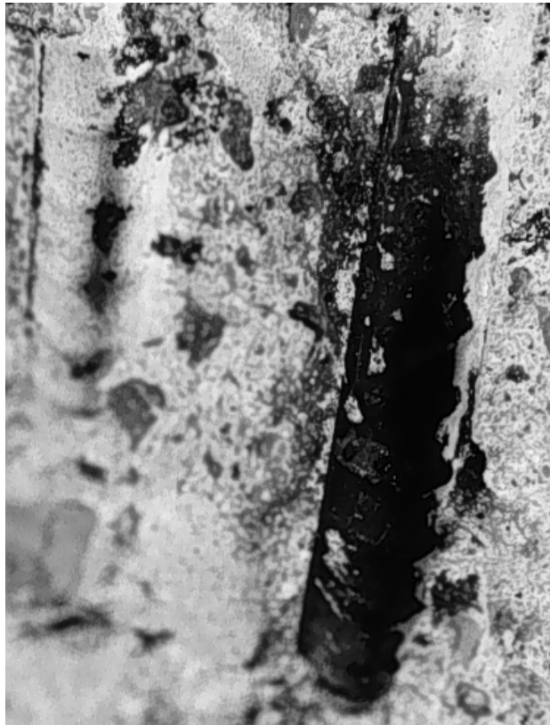
Figure 3.10 Stirrup trace in concrete adjacent to crack after one year.
