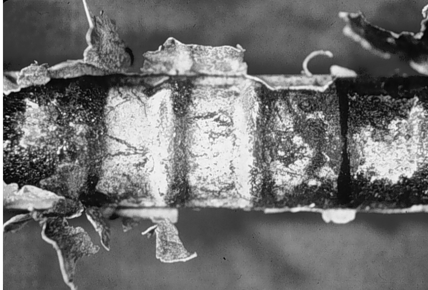
Figure 2.75 White residue of dried solution trapped beneath coating.
